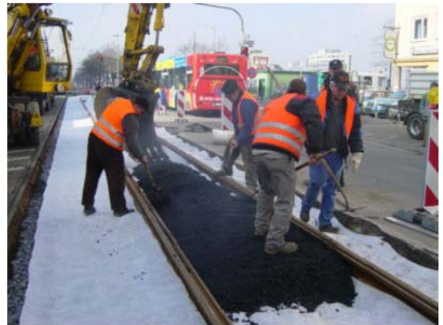
Frankfurt am Main: AC 32 T S 30/45, temperature reduced during manual paving at 3 °C outdoor temperature
